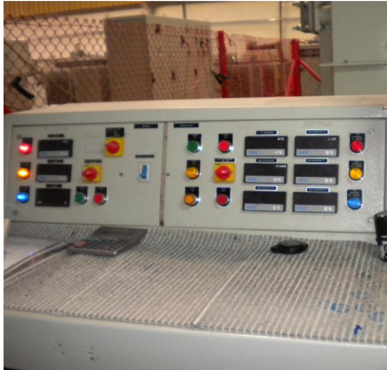
Fig 4.: Induced Over Potential Test Control Panel
