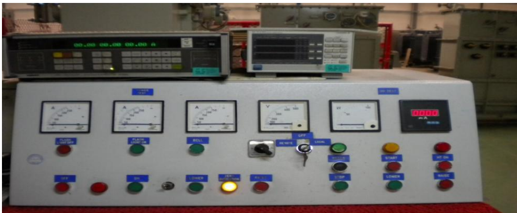
Fig 5 : No Load Loss Control Panel
